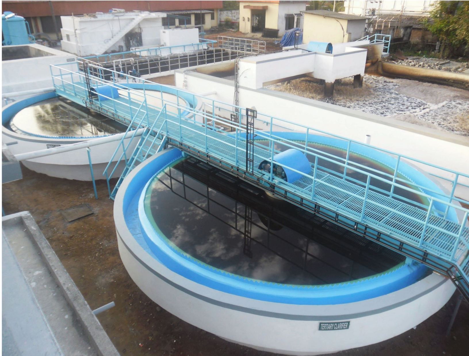
Clarifier Rake Mechanism @ Oushadhi Thrissur.
